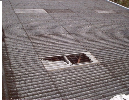
Short sheeting in poor condition
