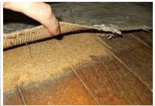
Contaminated carpet underlay
