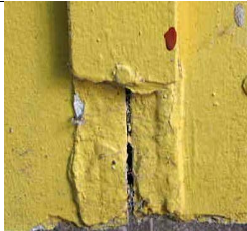
ACM batten (broken)
