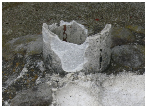
Broken ACM downpipe
