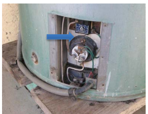
Cement millboard inside h/w system
