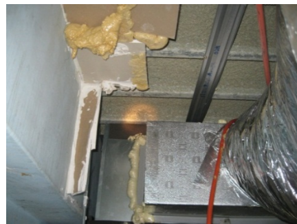
ACM as vermiculite over plasterboard
