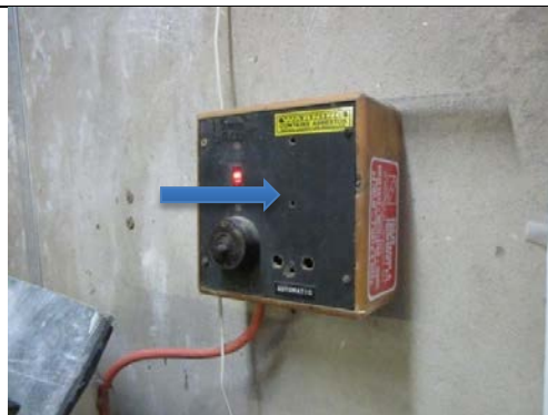
Cement sheet (black) fuse board
