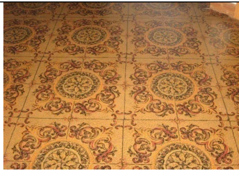
Linoleum with friable ACM backing
