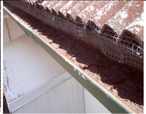
ACM debris in gutter from roof
